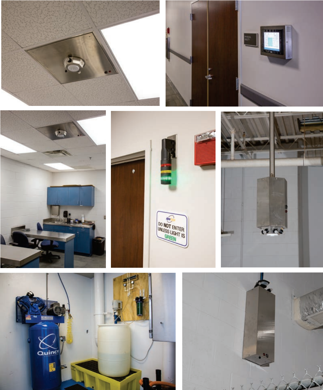
From top left: 1) Drop-in style hub replaces a ceiling tile in the gymnasium; 2) Touchscreen controller on the hallway wall; 3) Drop-in hub in Evidence Processing Room; 4) Warning light outside a treatment area; 5) Pole-mounted hub hung from the rafters in the Vehicle Bay; 6) AeroClave control room with equipment; 7) Wall-mounted hub in the K9 Kennel.
