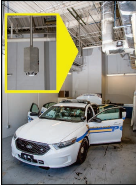
Vehicle Decontamination Area (Inset: Pole Mounted Hub)
