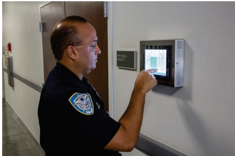
Hydra System touchscreen controller outside treatment area
